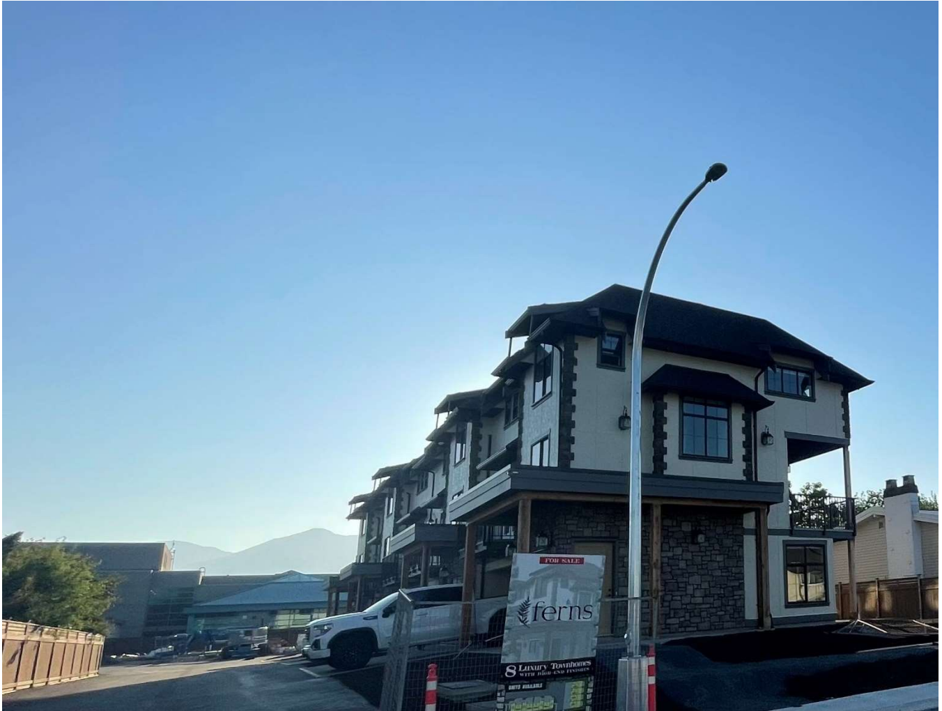
New 8-unit Townhouse Development two lots north of the property in question. 4 Units are almost complete and 4 units have foundations only.
